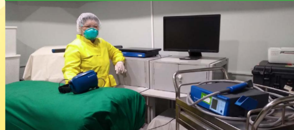
Engineering controls such as exhaust fans in all rooms, HEPA filters, UV light, sterilizers, barriers, taffeta covers for the equipment and PVC blinds that can easily be disinfected were installed.
